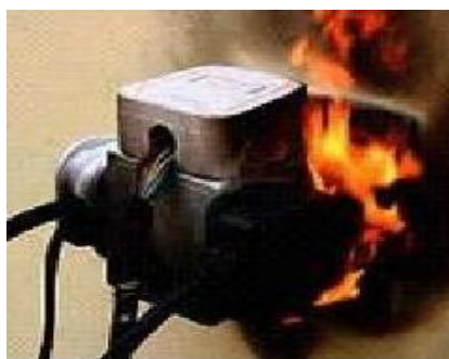
Fig 1.2: Fire in electrical appliances/equipment.
